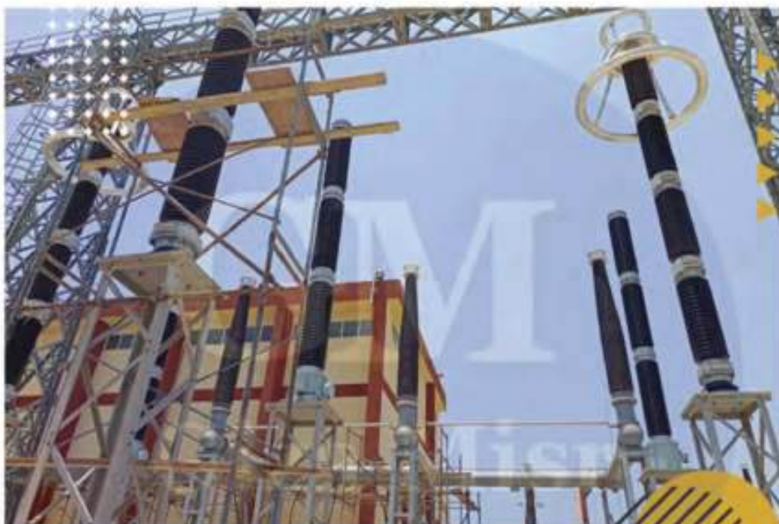
Substation Zagazig 500/220/66/11 KV
