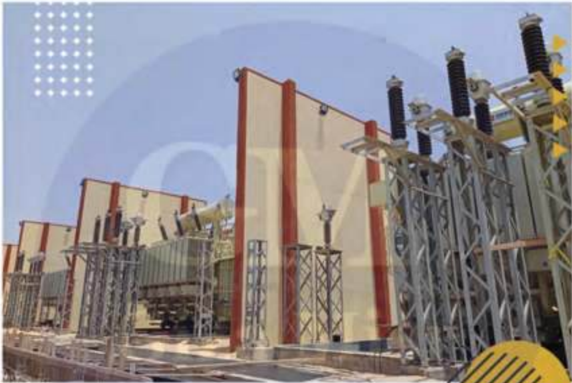
Substation Zagazig 500/220/66/11 KV
