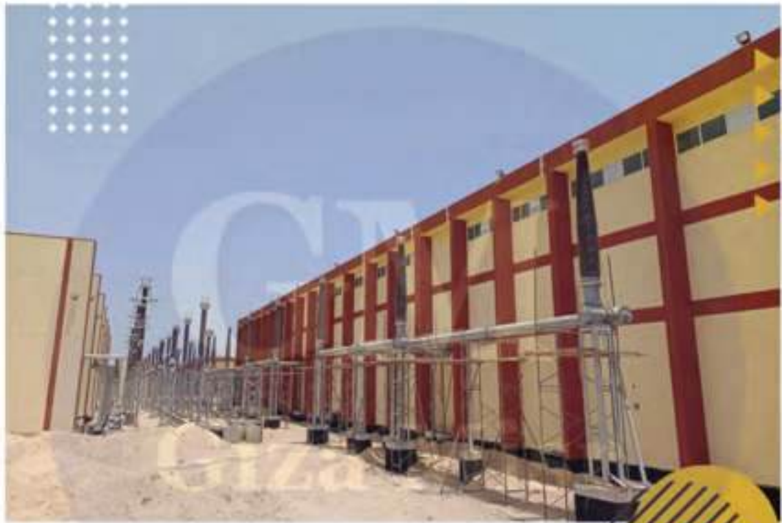
Substation Zagazig 500/220/66/11 KV
