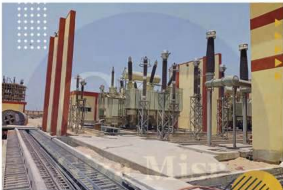
Substation Zagazig 500/220/66/11 KV
