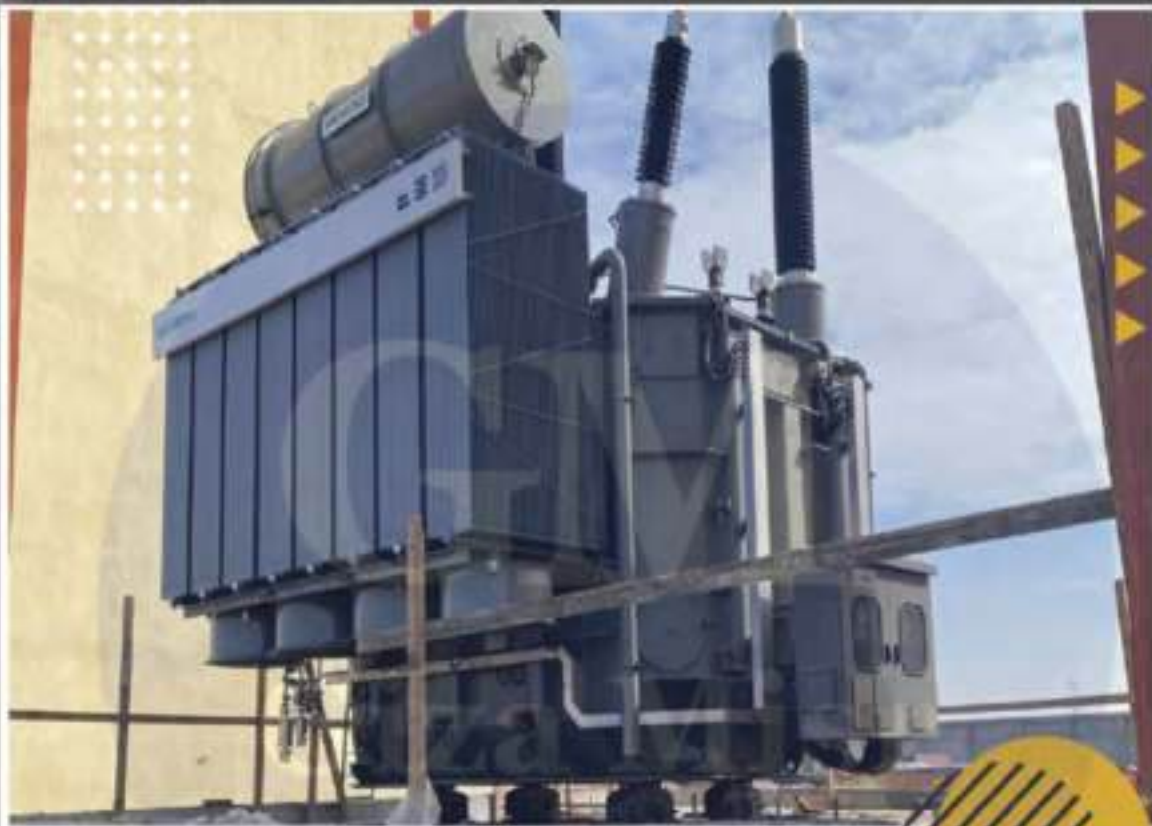
Substation Zagazig 500/220/66/11 kv
