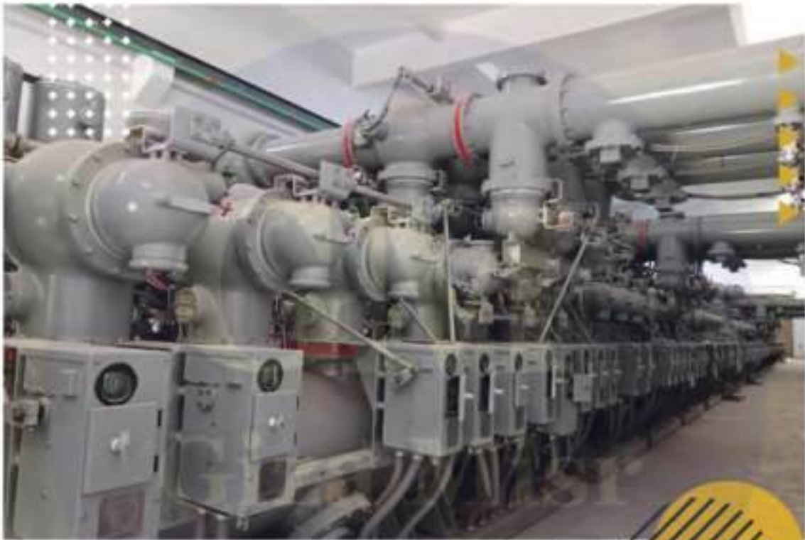
Substation Zagazig 500/220/66/11 KV
