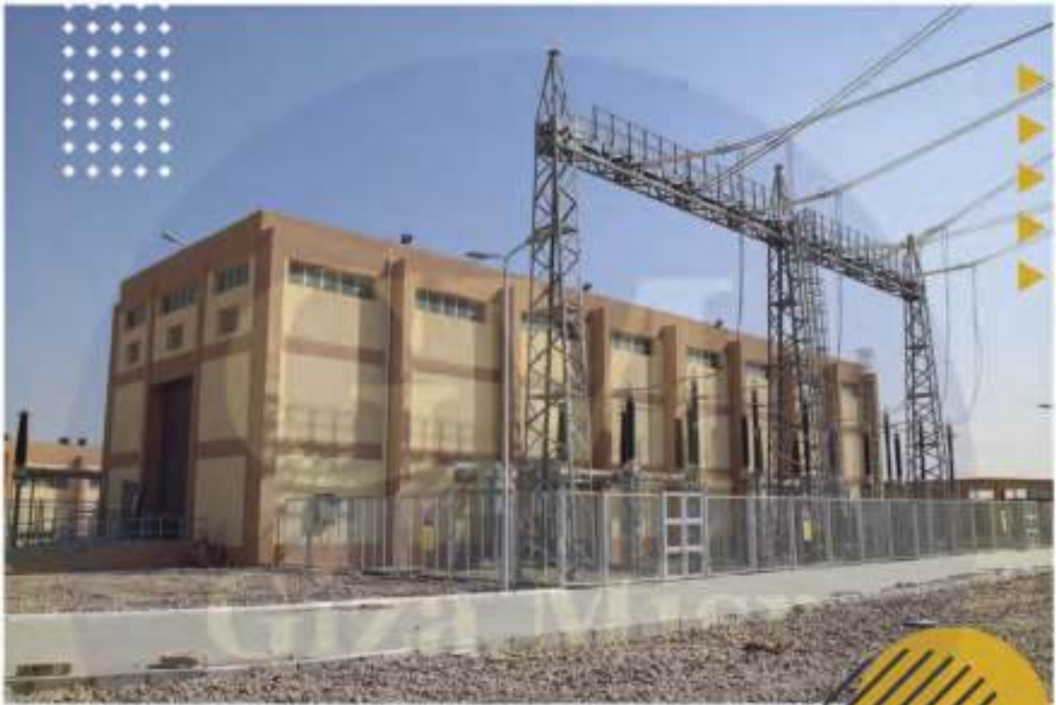
Substation West of El Shorouk 220/22/22 KV
