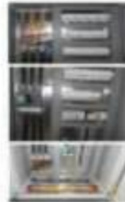
DC & AC Cabinet
