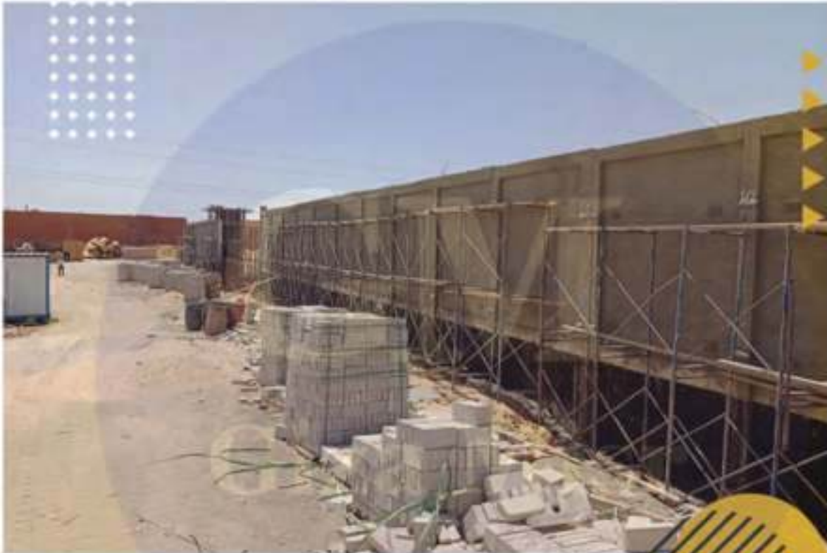
6th October Substation 220/22/22 KV
