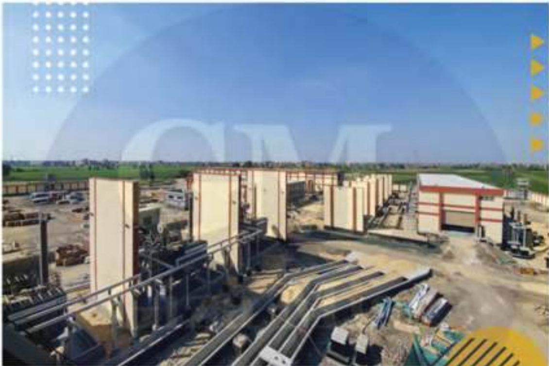
Substation Zagazig 500/220/66/11 KV
