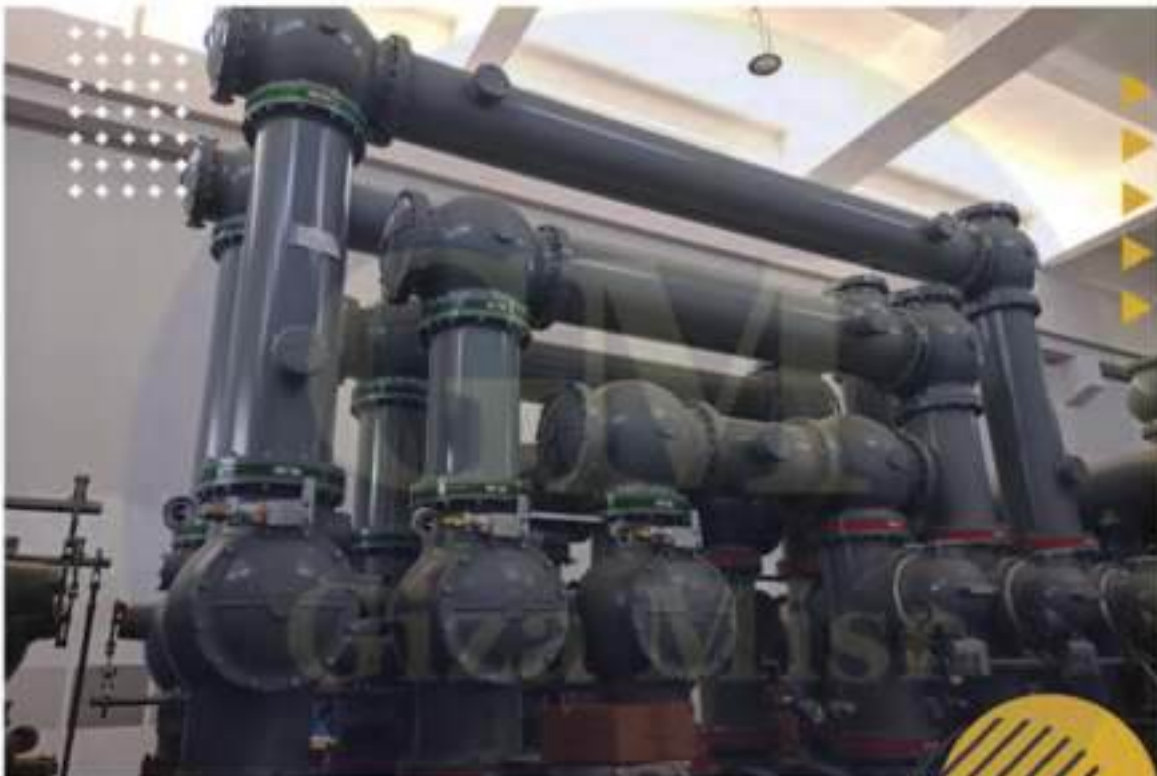
6th October Substation 220/22/22 KV
