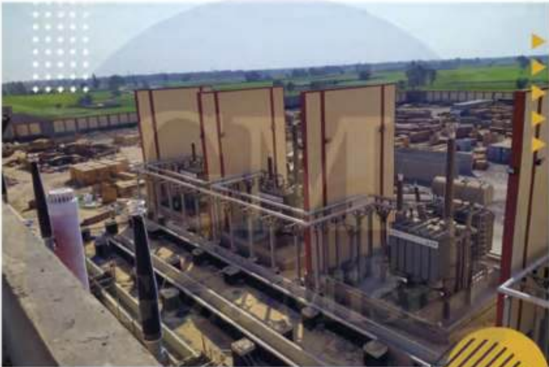
Substation Zagazig 500/220/66/11 KV
