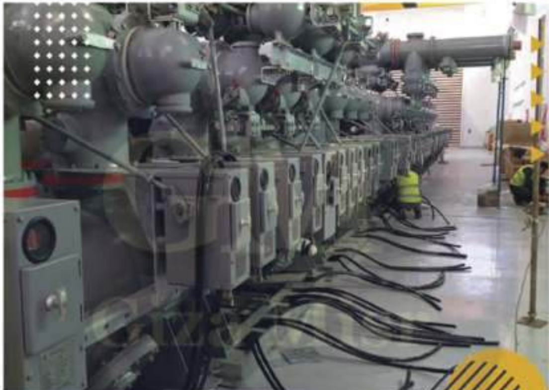
Substation Zagazig 500/220/66/11 kv
