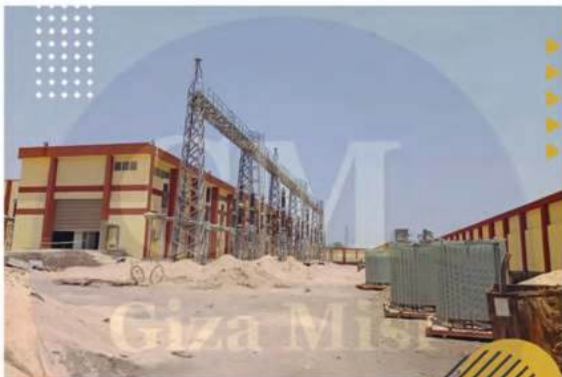
Substation Zagazig 500/220/66/11 KV
