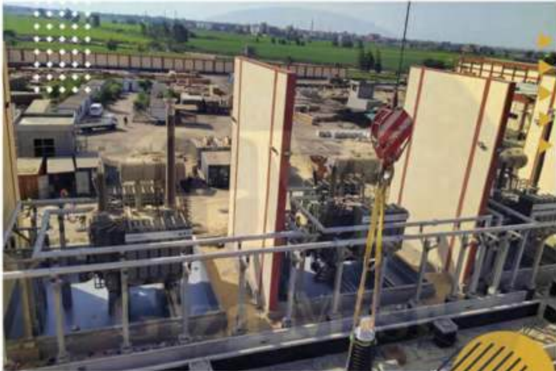
Substation Zagazig 500/220/66/11 KV
