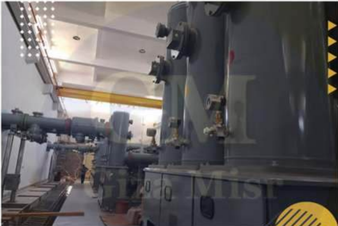
6th October Substation 220/22/22 KV
