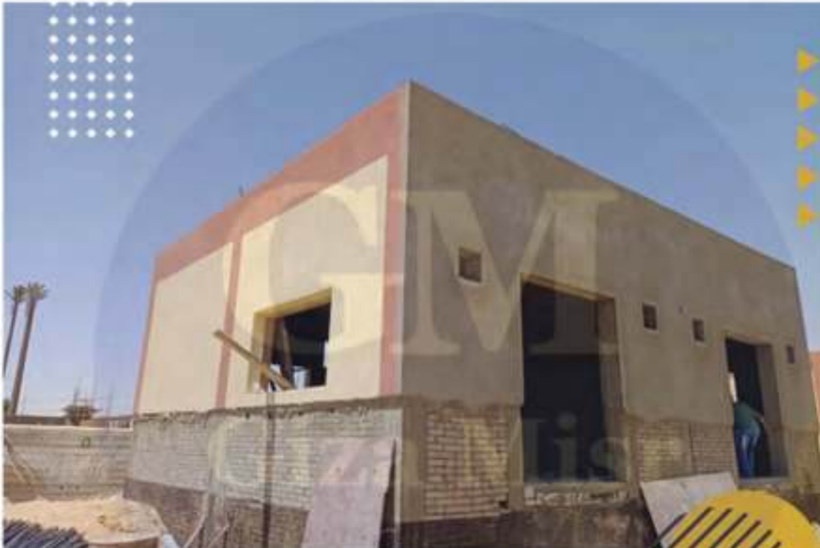
6th October Substation 220/22/22 KV
