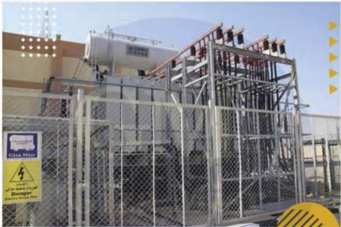
Substation West of El Shorouk 220/22/22 KV
