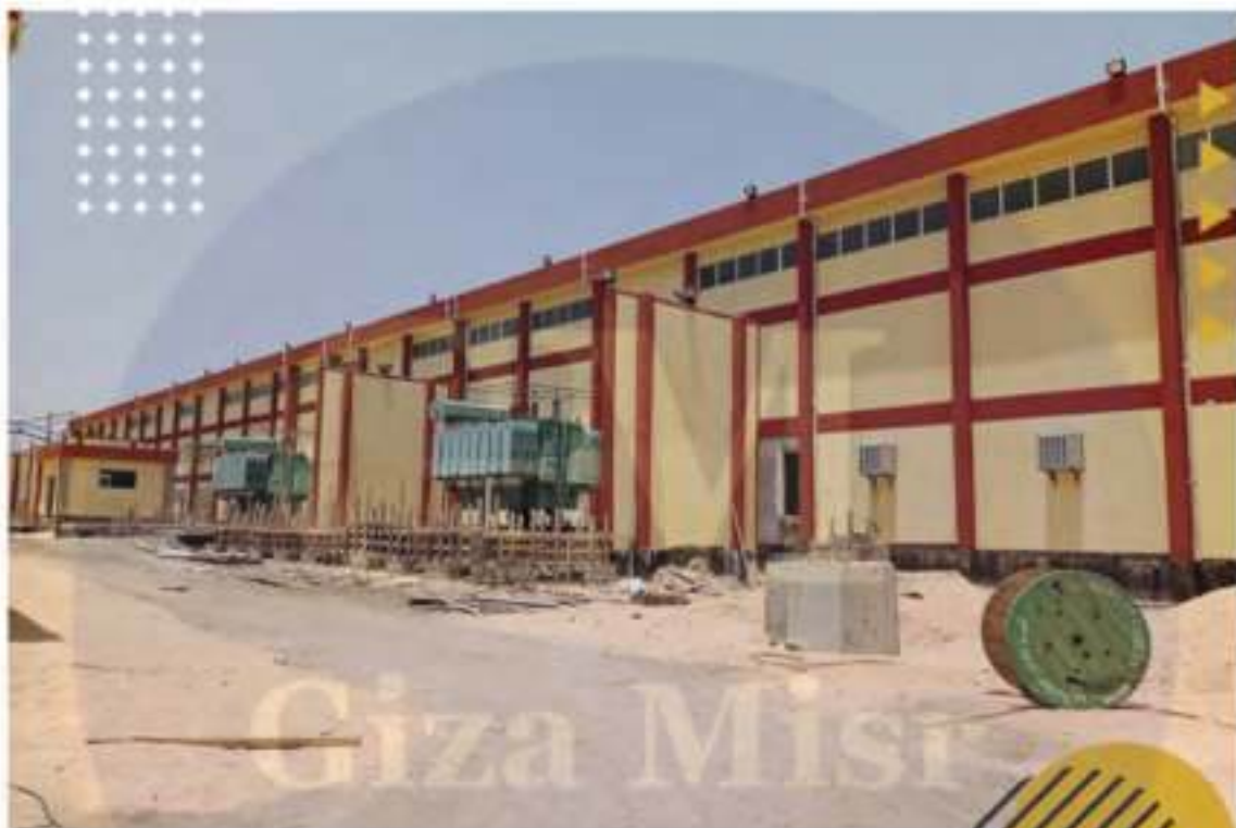
Substation Zagazig 500/220/66/11 KV
