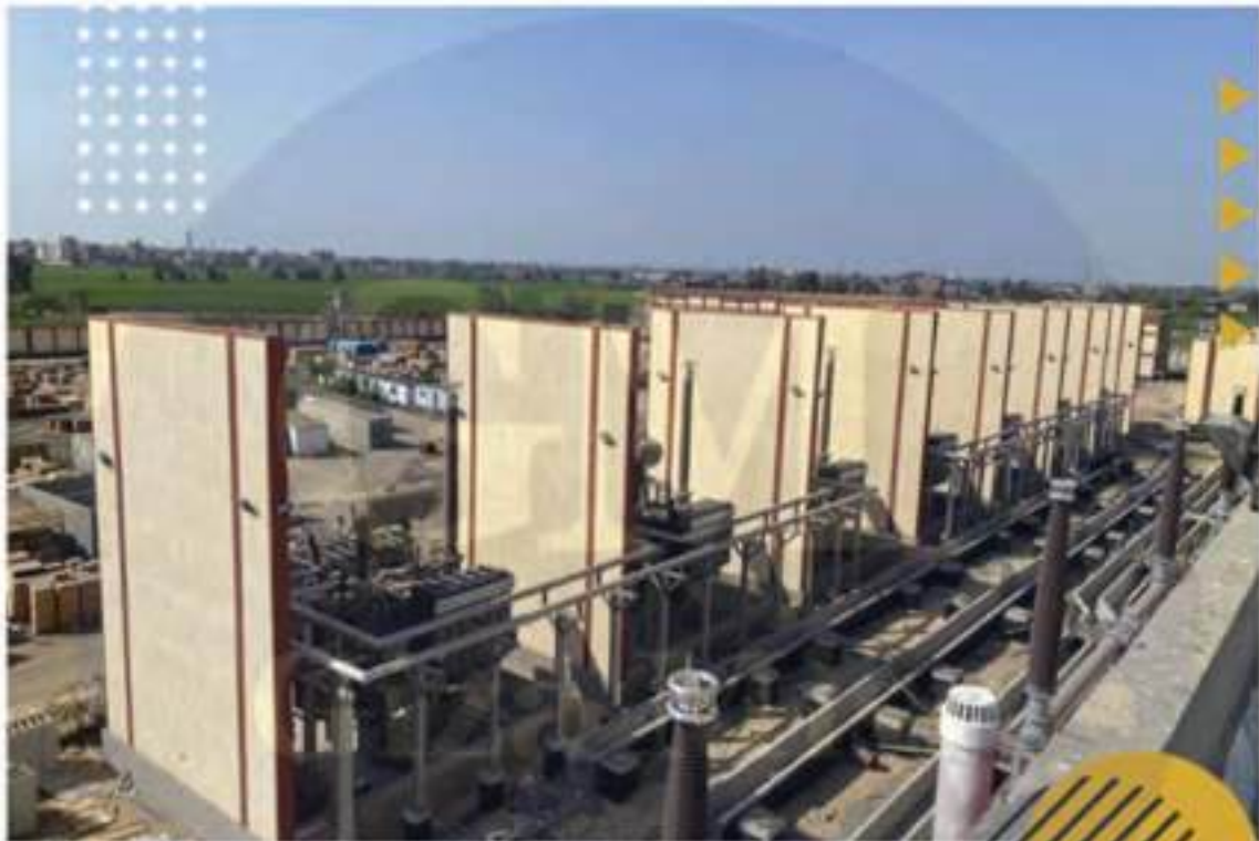
Substation Zagazig 500/220/66/11 KV
