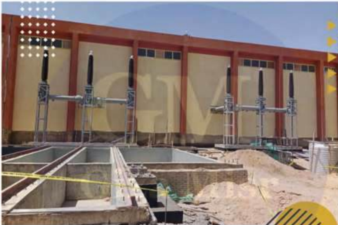
6th October Substation 220/22/22 KV
