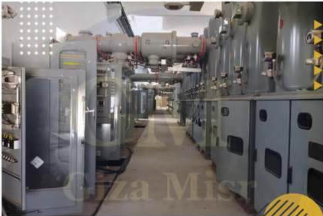
Substation Zagazig 500/220/66/11 KV
